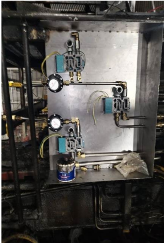
Panel is installed where indicated by plant
